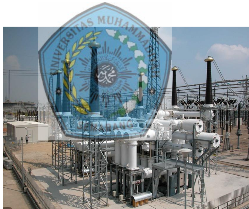
Gambar 1. Gas Insulated Substation (GIS)
