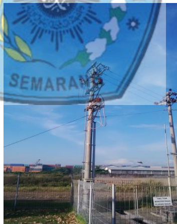
Gambar 2.6. Gardu Distribusi Terminal LPG Semarang
